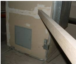
AHU-1 Relief Fan RF-2; Note access through hatch to fan. RF discharges to hanger space through grille on right side of rated enclosure. RF-1 the same about 6 feet behind.
