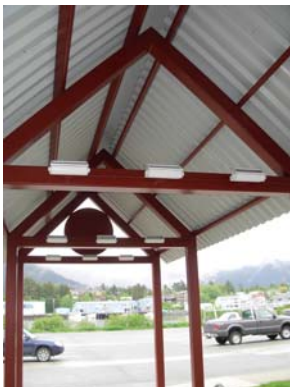
Fig 8: Entrance Canopy Lighting
