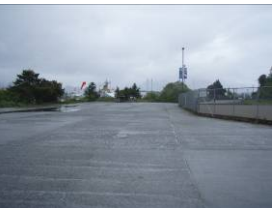
Undefined access road
