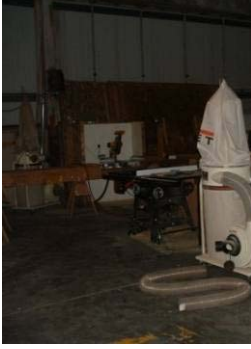
Dust Collection System
