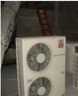
AC-1 & AC-2 Condenser Units rejecting heat to Hangar open space.
