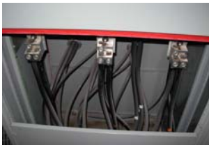
Fig. 3: Main Switchboard Service Entrance
