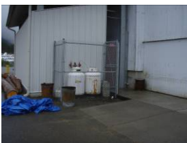
Propane Tank Storage
