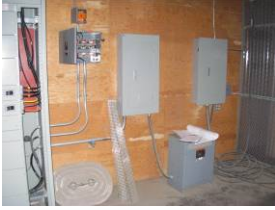
Fig. 4: Panelboards & Step Down Transformer
