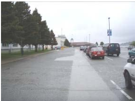
Pavement with patch for sewer
