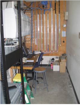
Figure 11 - Telephone Terminal Board and Switch
