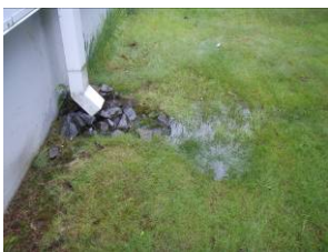
Standing water at building
