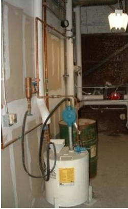
Chiller Circulation Pump and Glycol Fill Station.
