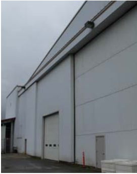
Fig. 7:Exterior Wall-mounted Luminaires
