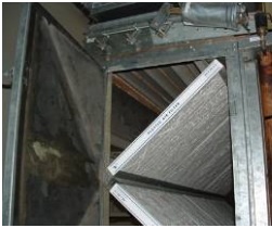
Inside AHU-1 looking at mixing box. Note corrosion of dampers and deteriorating insulation liner.
