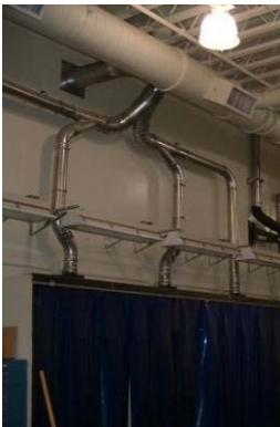
WELDING BOOTHS EXHAUST AIR MANIFOLD, ARM
