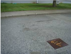
Embedded steel in pavement and lid of derelict fuel vault
