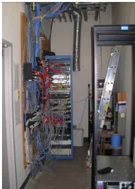
Fig 12: Network Rack and Distribution System
