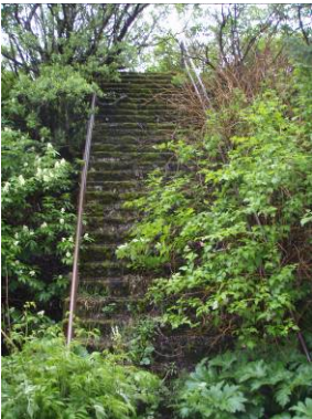
Derelict stairs at South Side of building
