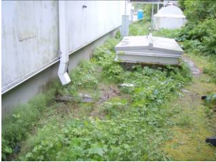
Rain leader & derelict vault
