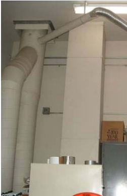
AHU-1 SUPPLY DUCT WITH MODIFICATIONS – NOTE SMALL DUCT ADDED
